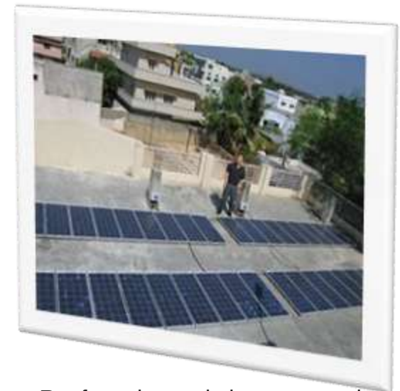
Rooftop photovoltaic power station
