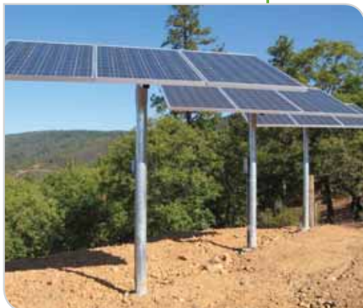
> 4.5 MW off-grid installation (California, USA)
