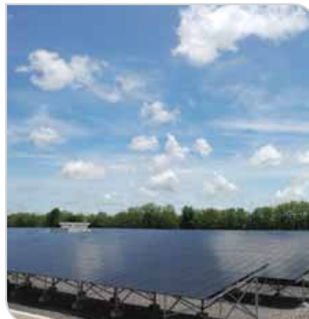
> 7.5 MW power plant (Phetchabun, Thailand)
