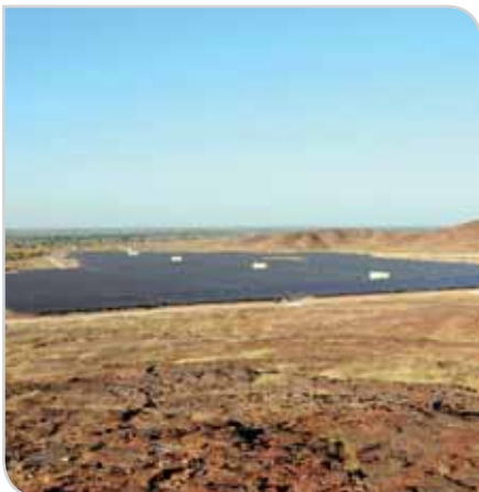
> 5 MW power plant (Osiyan, India)
