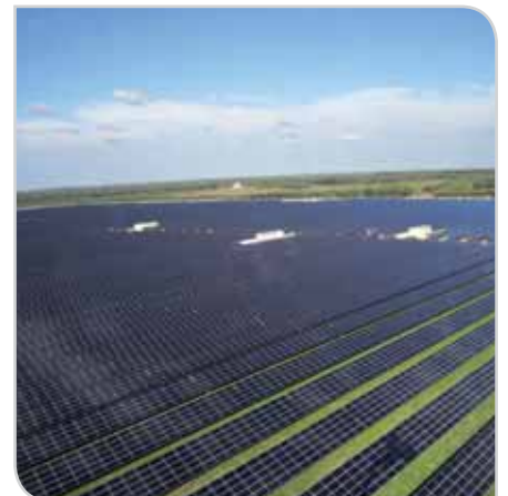
> 43 MW power plant (Plugia, Italy)
