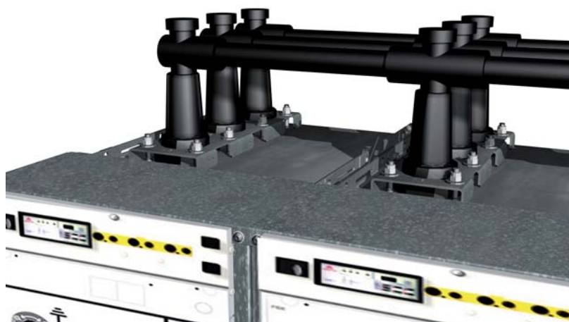
View of the busbars
