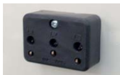
VPIS, Voltage Presence Indicator System
