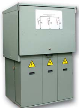
Flusarc 36 outdoor switchgear with front hatch closed
