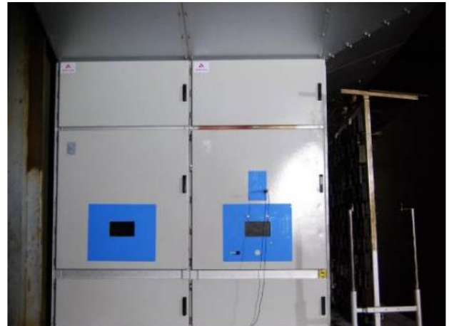
DNF7 before internal arc test at STL laboratory
