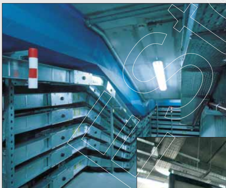
Example of a busbar installed in confined spaces
