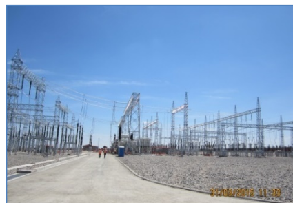
S.E. San José 500/220 kV
