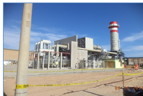
Turbina a gas (TG2)
