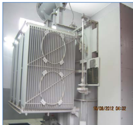
Transformador Principal 17/20 MVA 13,8/22,9 kV
