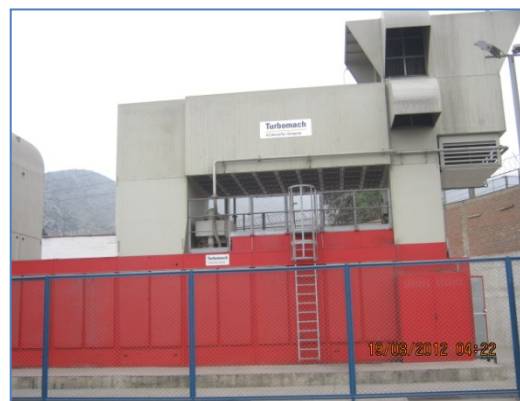
Turbina a Gas
