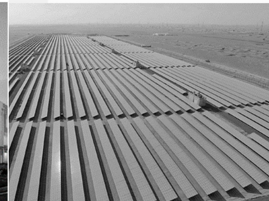
DEWA PV 260 KW Power Plant Dubai
