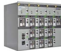
Power distribution and circuit protection
