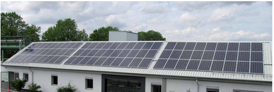
Figure 13: Solar power system
