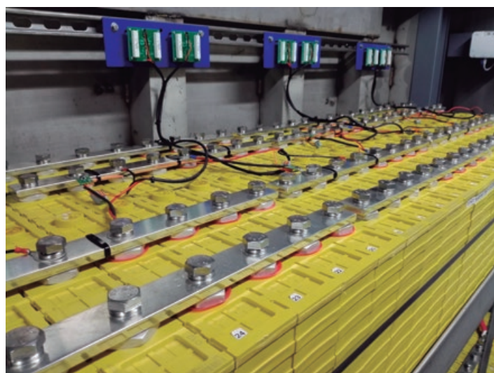
Figura 2. Sistema de baterias [Yo-Co-Man / CC BY-SA] ( https://creativecommons.org/licenses/by-sa/4.0/ )
