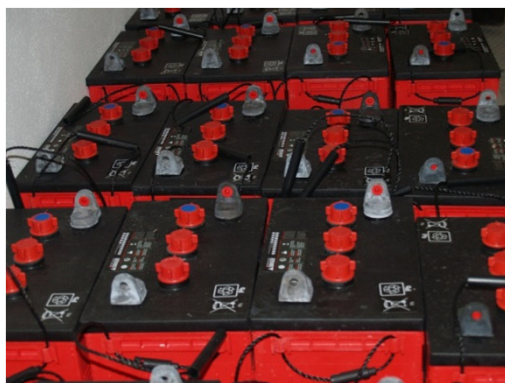
25 kWh Flooded Lead-Acid (FLA)
