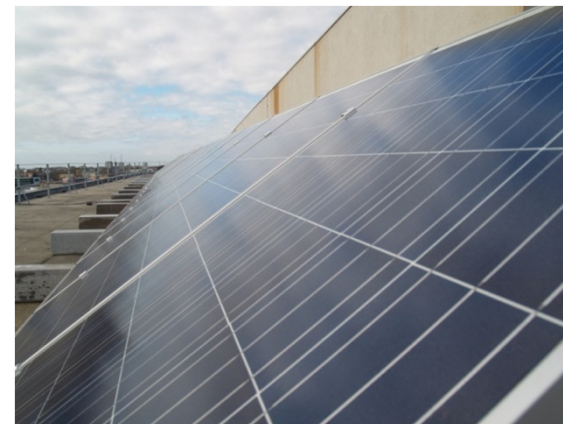
15 kWp photovoltaic panels
