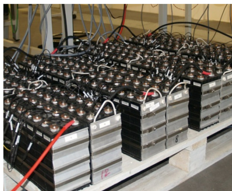
128 Lithium battery cells
