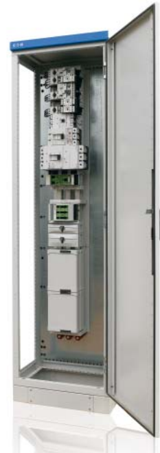
xVtl control distribution board
