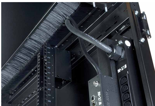
RP Series rack with 2 installed Eaton ePDUs
