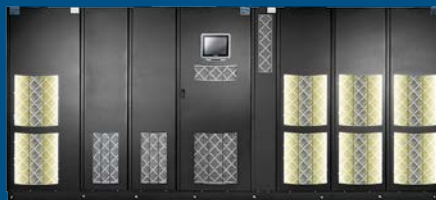
9395P on batteries
