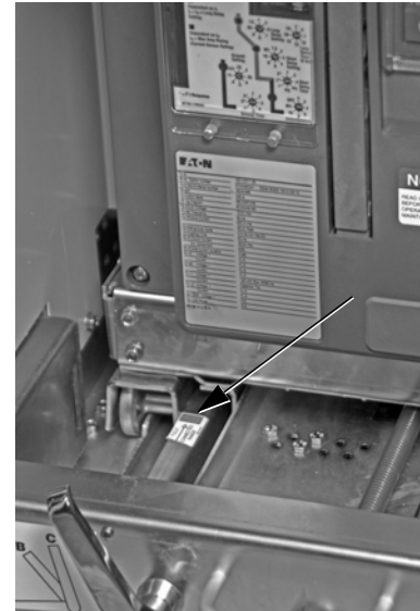
Circuit Breaker in Connected Position Indicator
