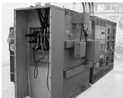
VFI with Secondary Unit Substation
