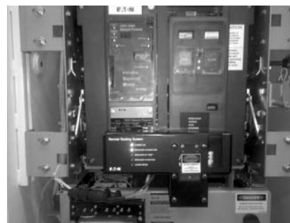
Remote Racking System
