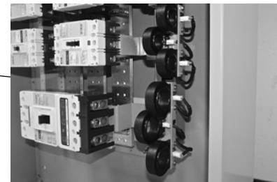
Pow-R-Line MPM—CTs are Factory-Mounted and Wired to Meter
