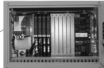
Factory Assembled and Wired Meters
