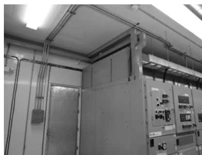
Arc Resistant Switchgear Inside IPA
