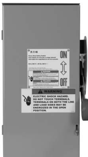
Solar Disconnect Switch
