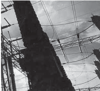
Bushing Power Factor, Partial Discharge and Vibro-Acoustics
