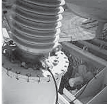
Online Transformer Insulation Monitoring System
