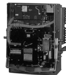
Reconditioned and retrofitted with new trip system.
