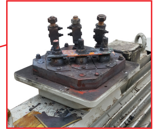
Contact resistance fault
