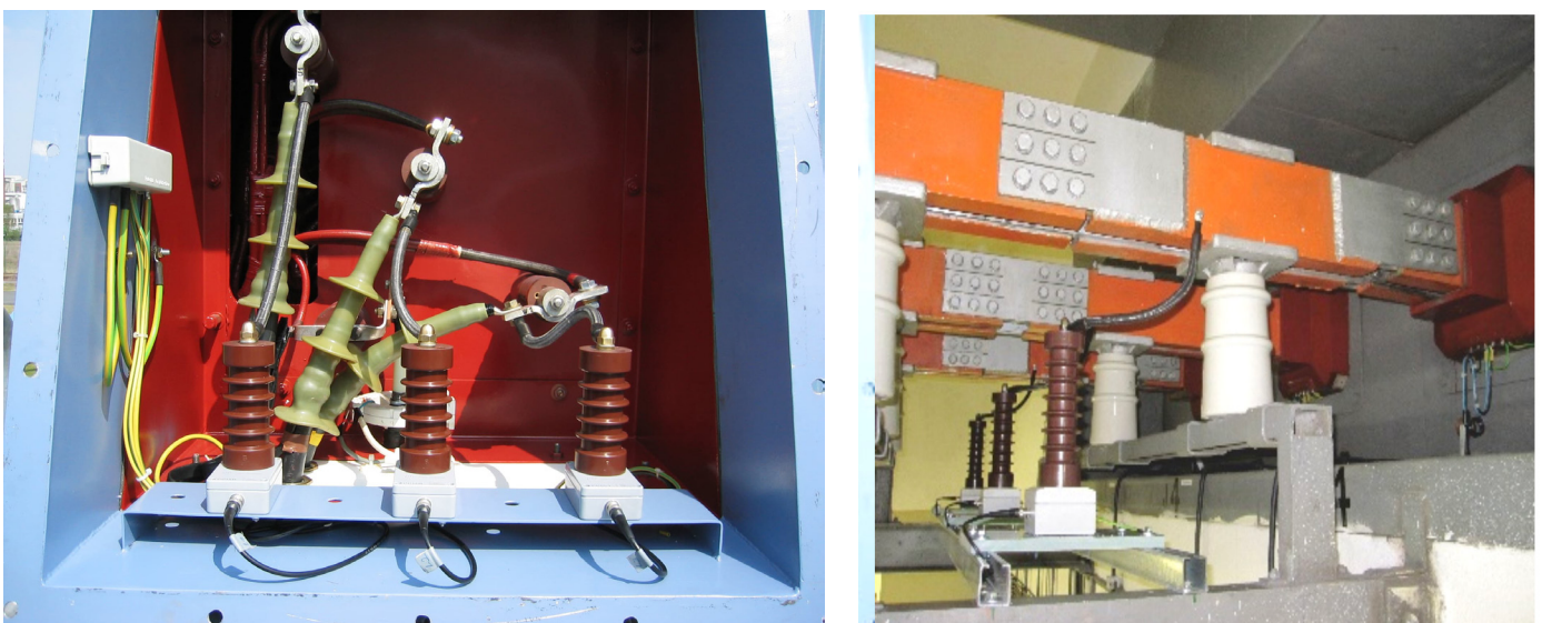
Figure 5. Example of preinstalled coupling capacitors on motor terminals (left) and on generator bus bars (right)
