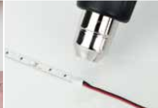
Non IP Rated LED strip connections heat sealed
