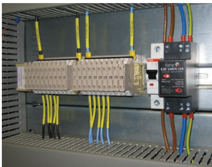
Figure 6. ESP240 DS-32A installed conveniently in a power distribution cabinet.
