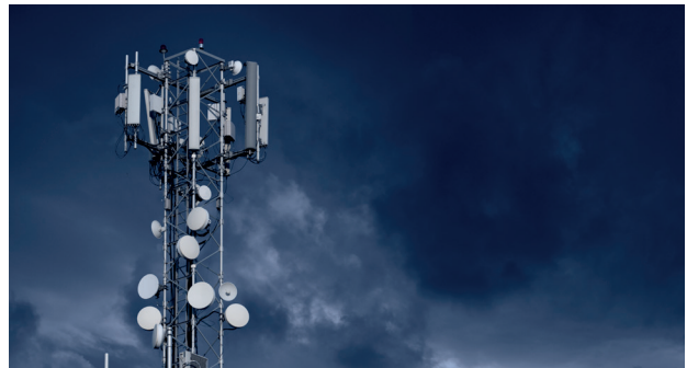
Telecom and Data
